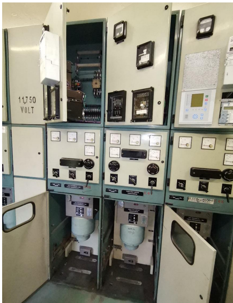
Figure 13: Old oil circuit breaker MV switchgear
