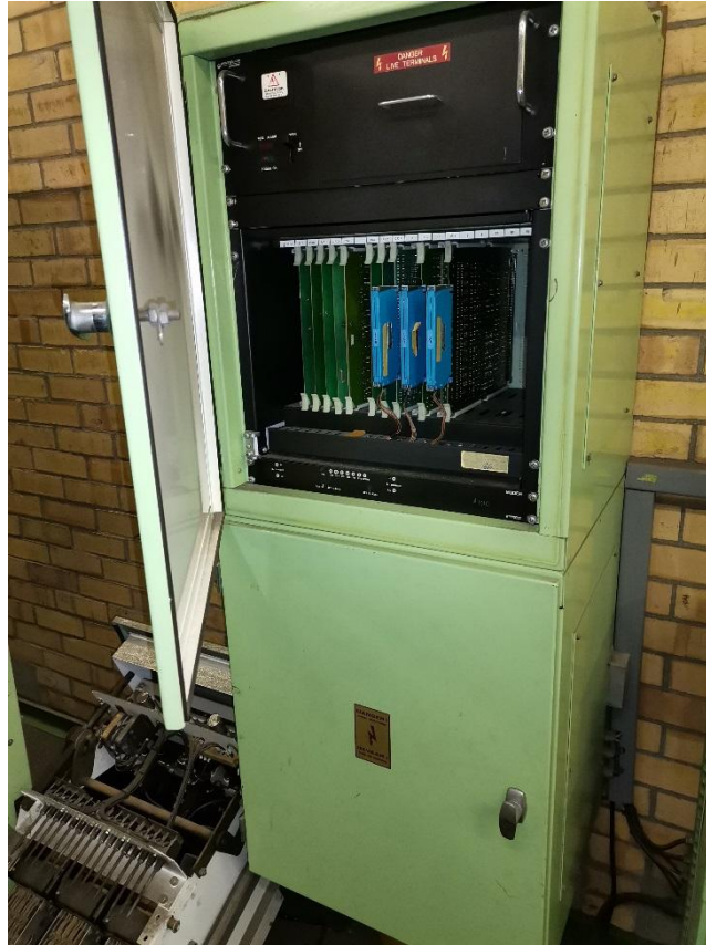
Figure 15: SCADA instrumentation board
