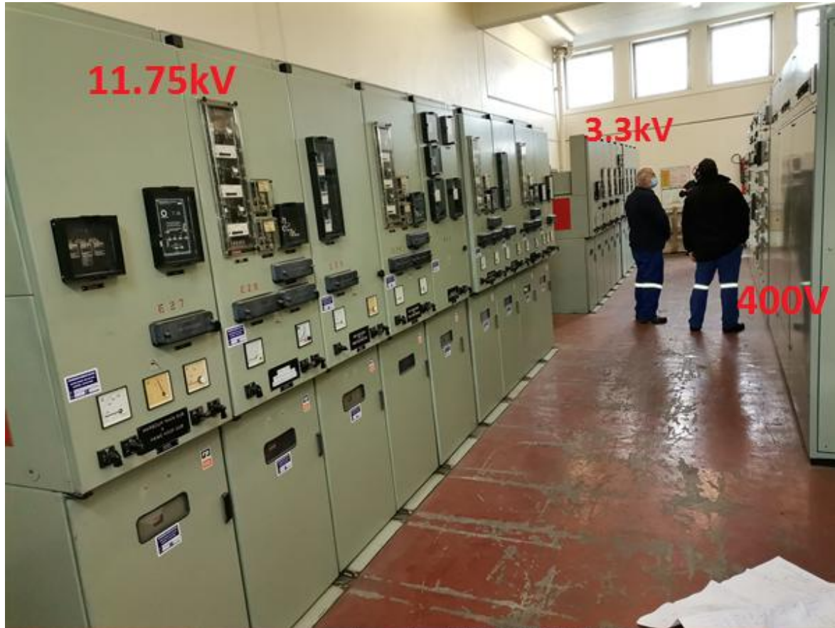
Figure 17: MV and LV Switchgear all in one room with no barrier in-between.
