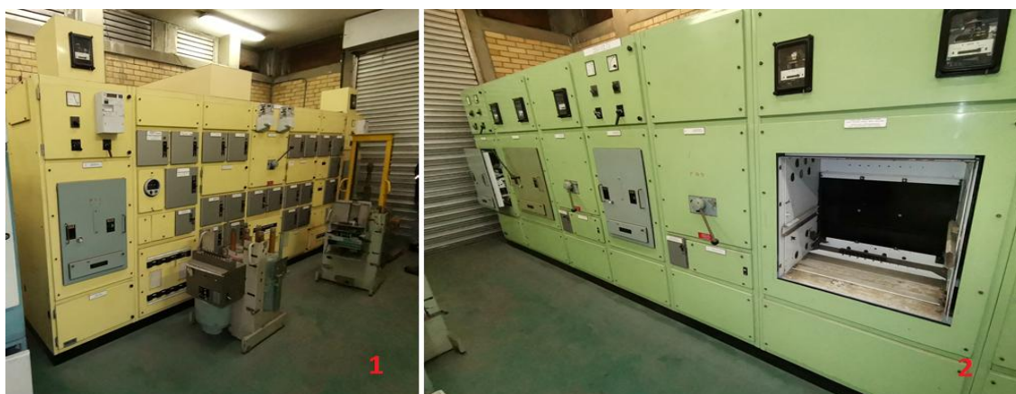
Figure 14: 400V and 550V switchgear
