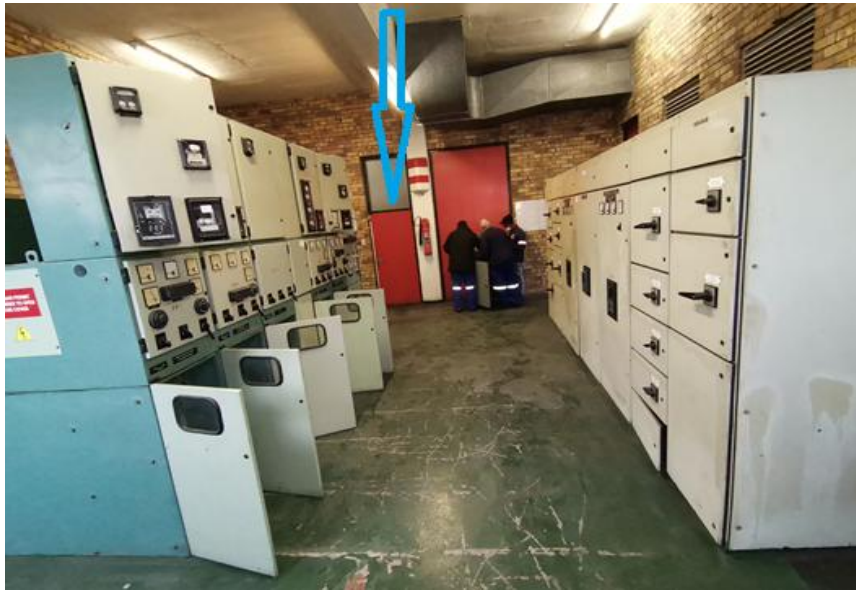
Figure 23: MV and LV Switchgear in one room with no barrier in-between.
