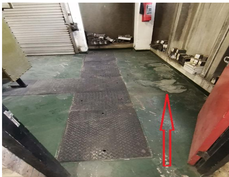
Figure 24: Transformer Room Roof Leak Stain
