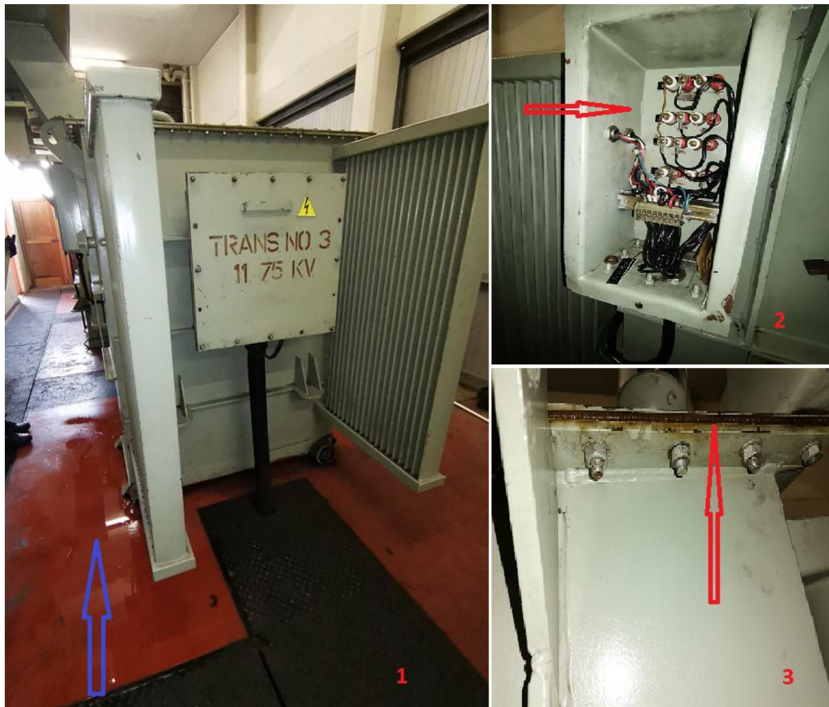
Figure 21,1 TRF Oil Leakage of the Floor. 2, TRF Auxiliaries with Oil Leaks. 3, Tank Seal with Oil Leaks
