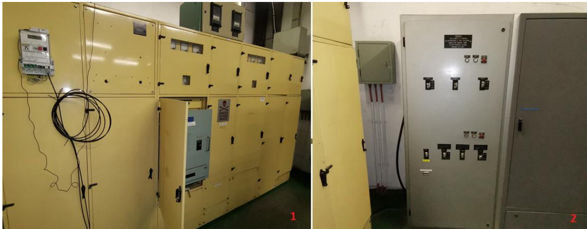
Figure 8: Old LV switchgear.
