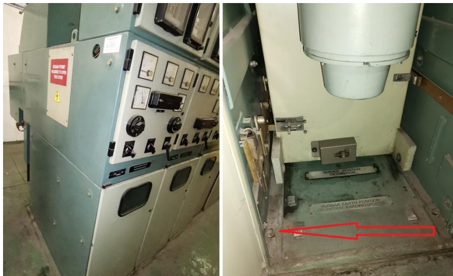
Figure 7: Old oil circuit breaker MV switchgear
