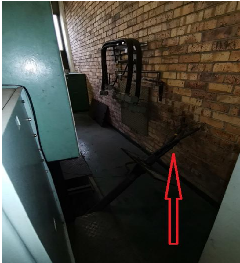
Figure 27: Faulty MV Incomer Cable Disconnected
