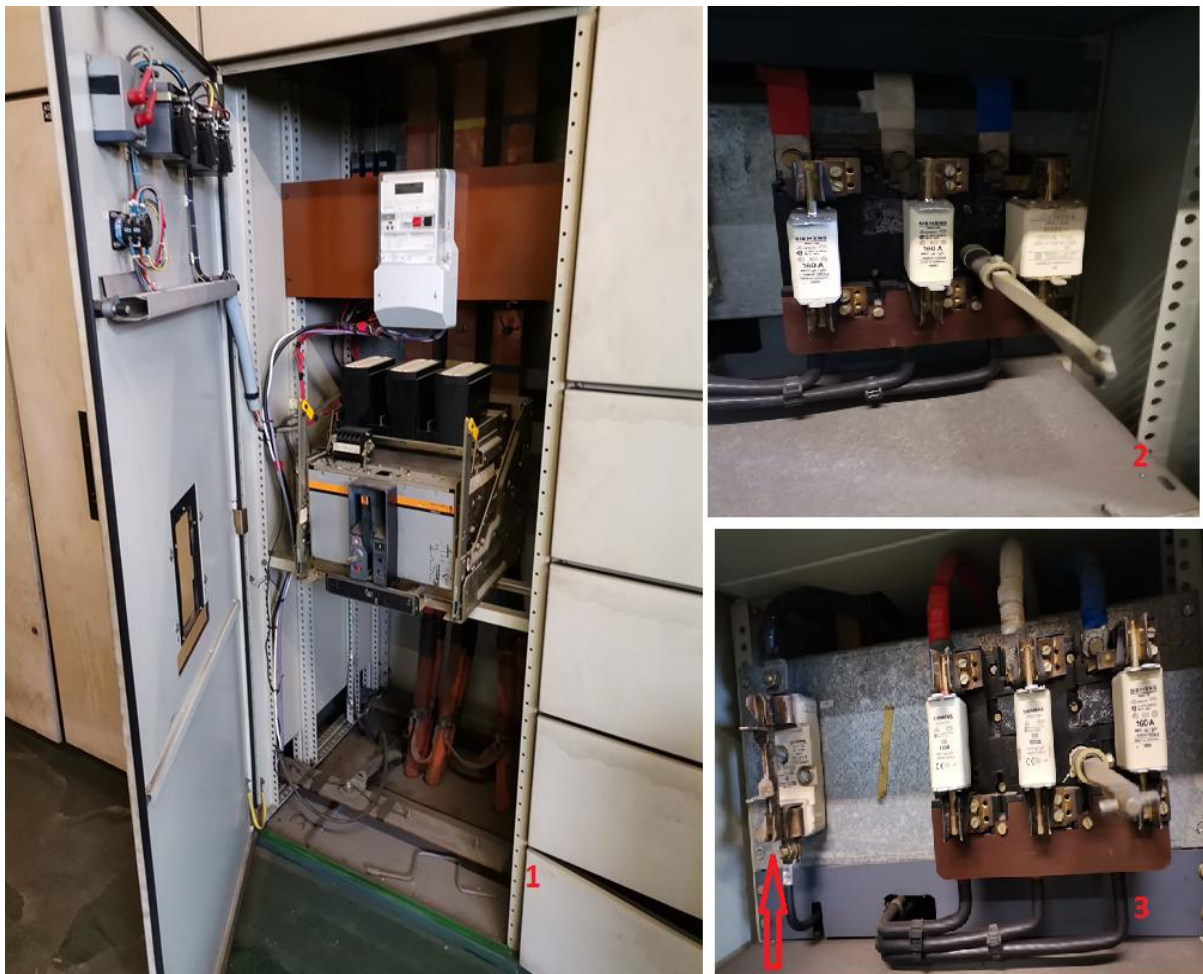
Figure 25: 400V Switchgear with (1) breakers and (2&3) details of the fuses
