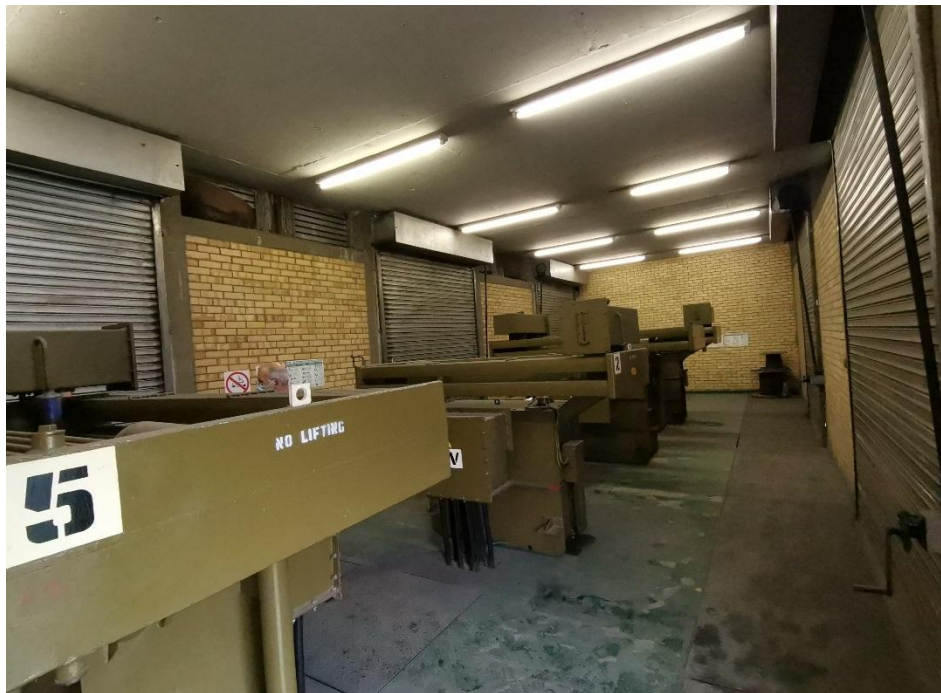
Figure 12: Distribution transformers with no oil containment provision.
