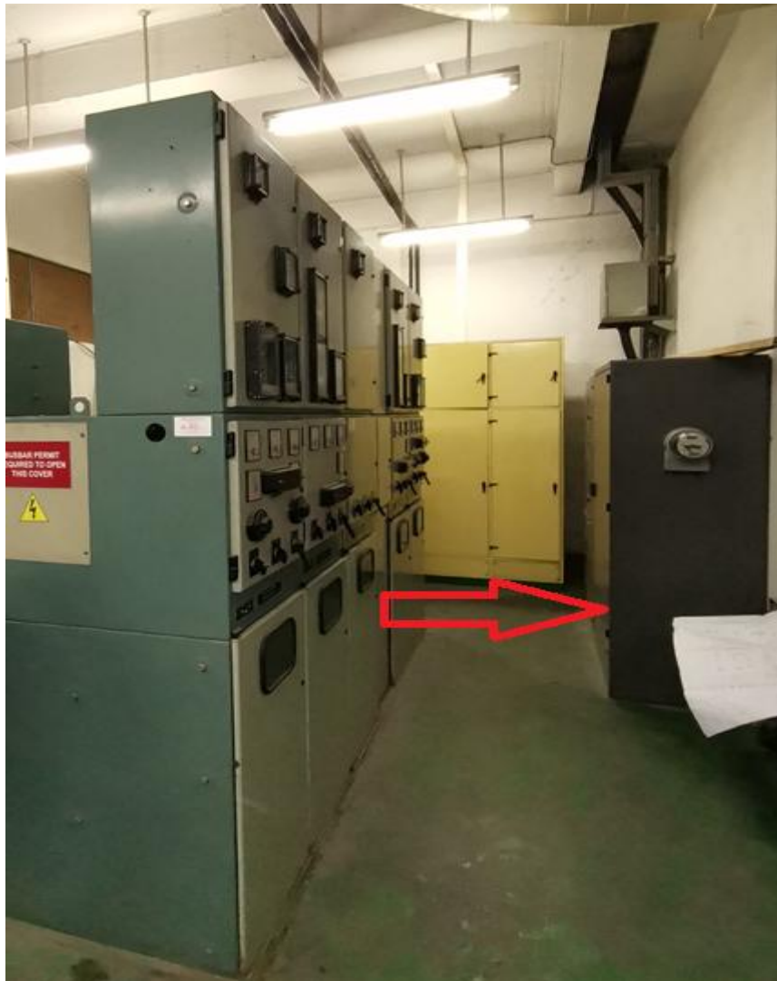
Figure 2: Racking space in front of the MV panel is less than 1200mm. MV switch gear is not separated by any form of barrier from the LV switchgear.
