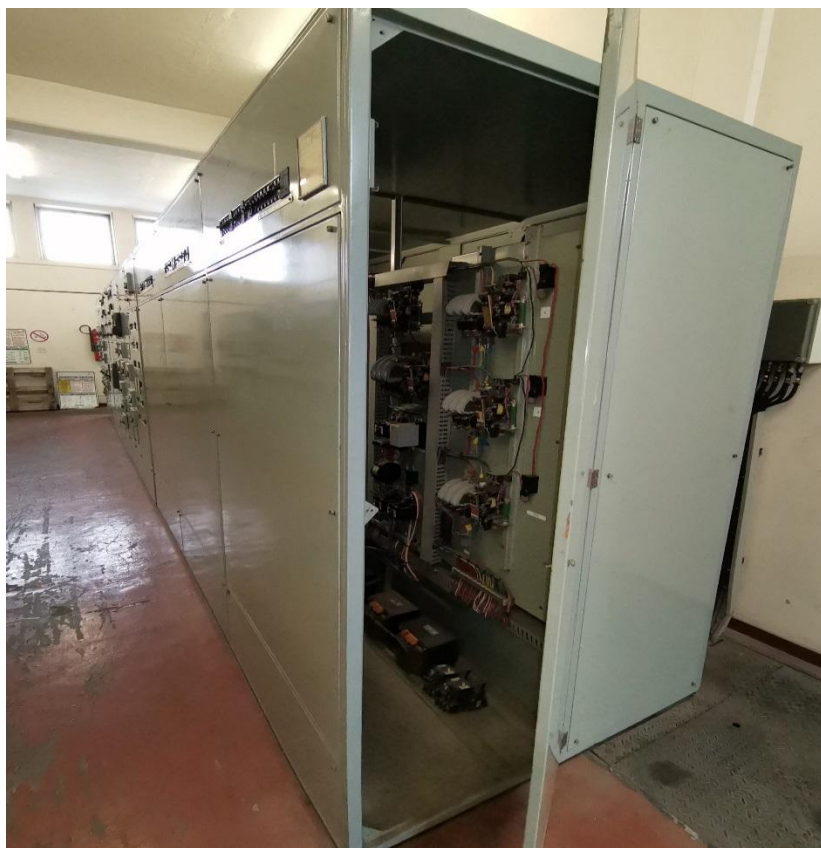
Figure 19: 400V Switchgear with a door opening on the side.
