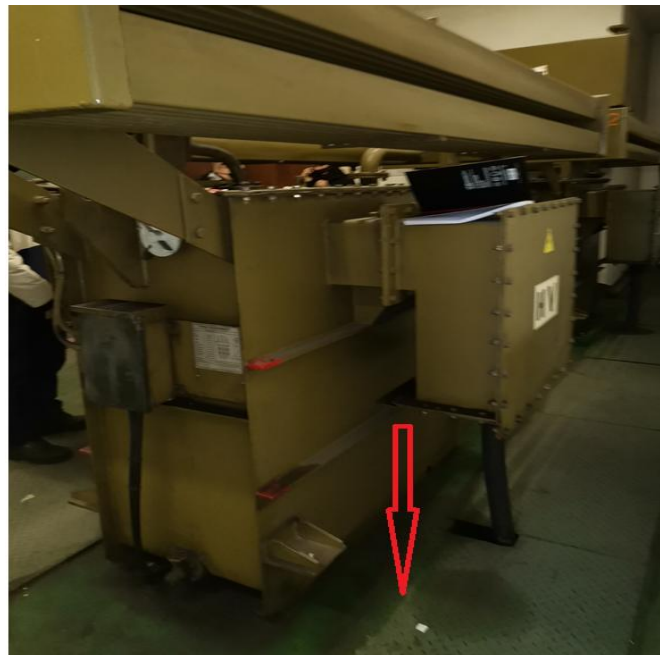
Figure 6: Distribution transformer with no oil containment provision.
