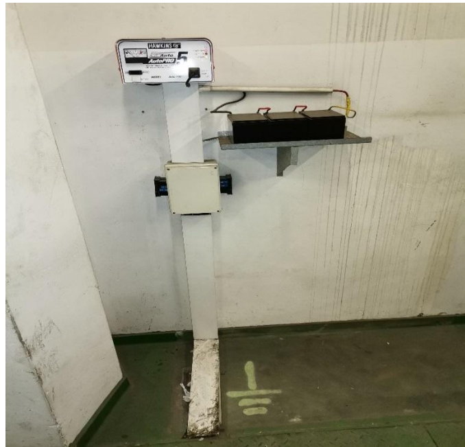
Figure 5: BTU with only three batteries.
