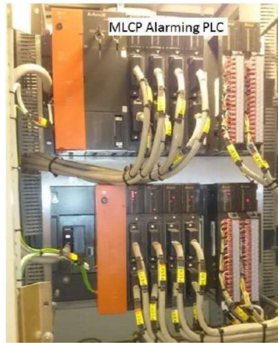
Photograph 42: MLCP Alarming PLC
