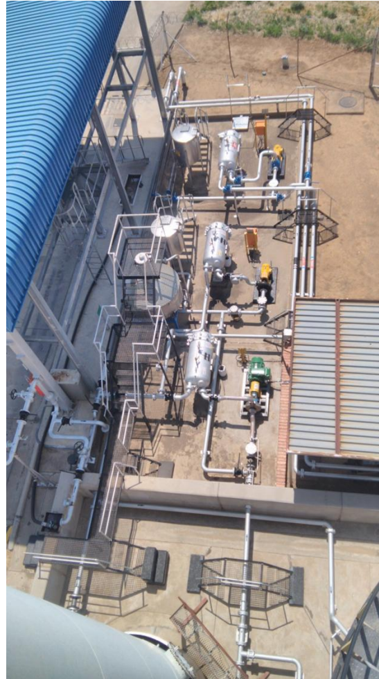
BFIA – Filtration Station
