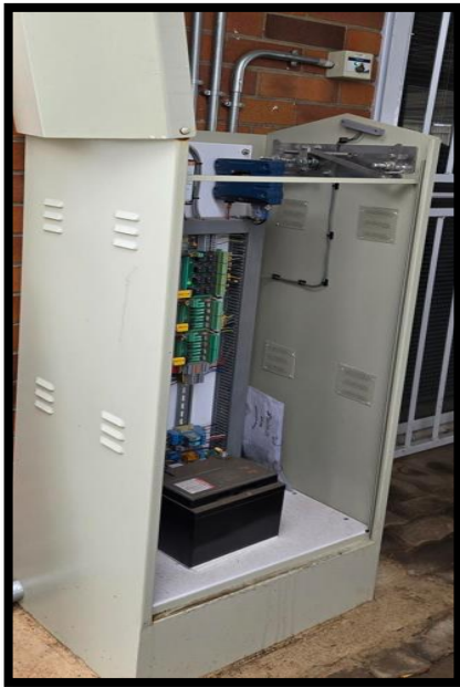
Figure 3 - Typical Compact Telemetry Enclosure as used on Sanitation Pump Station sites
