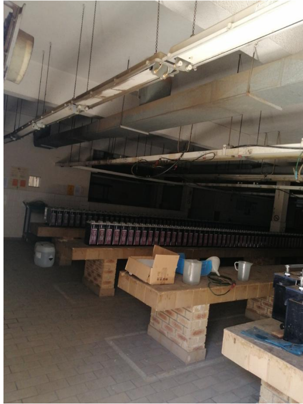
Figure 3: Photo of the Battery rooms
