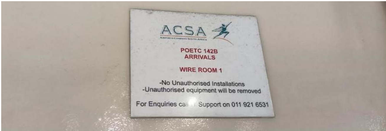
Figure 8: Wire Centre to which network cables for Booths # 11& 12 are connected.
