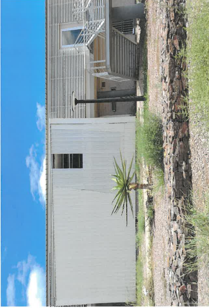
d) Damaged fibre glass sheeting
