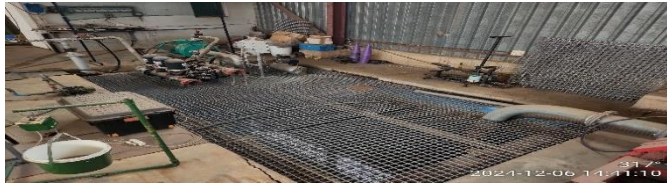
Figure 2: Picture of the existing underground 20,000-litre water reservoir inside the building
