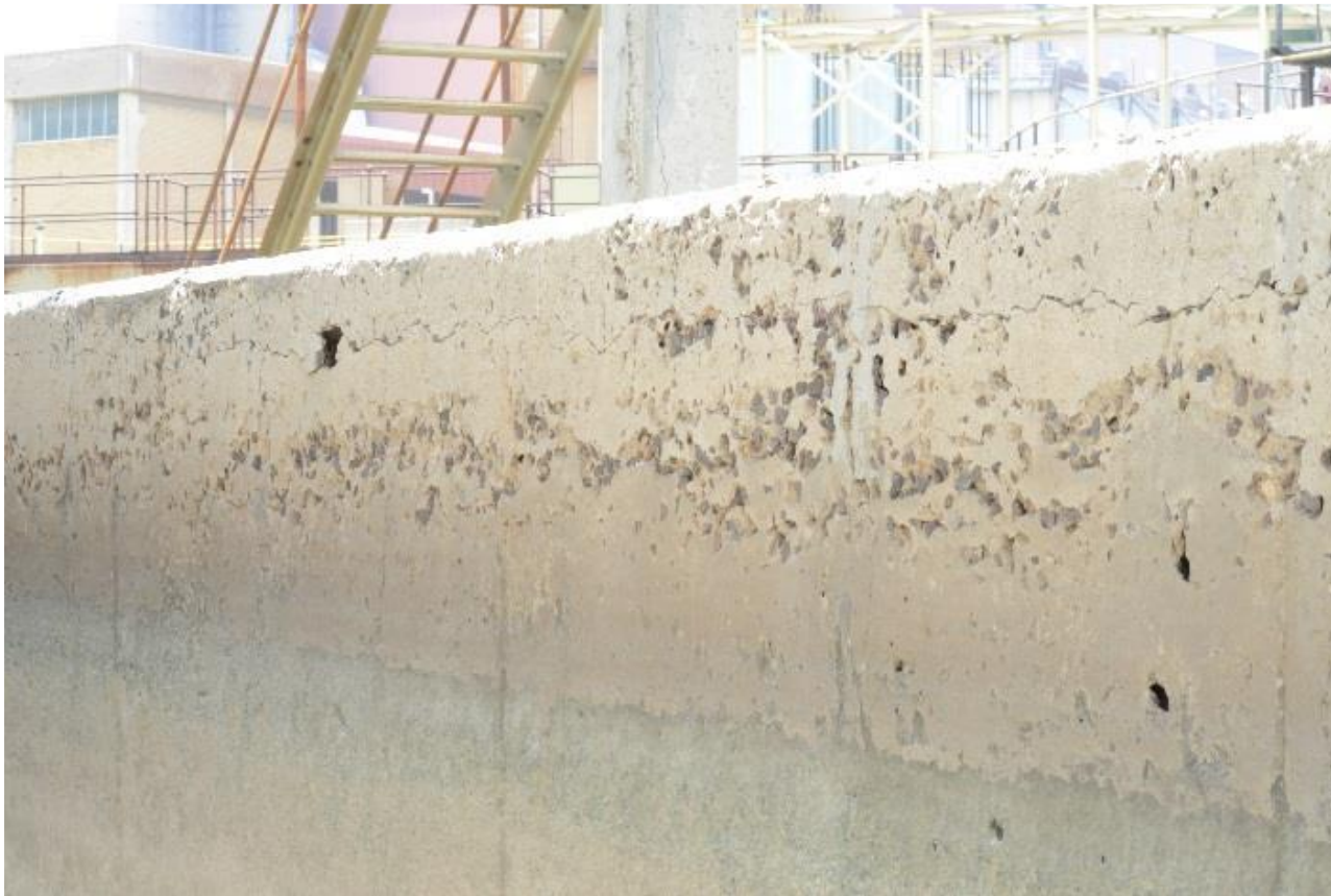
Figure 7: Pond internal walls cracking.
