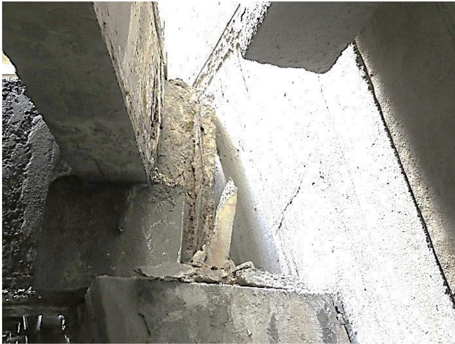
Figure 5: Cracking and spalling at beam corbel connection
