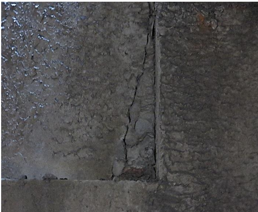
Figure 3: Cracking at beam edge
