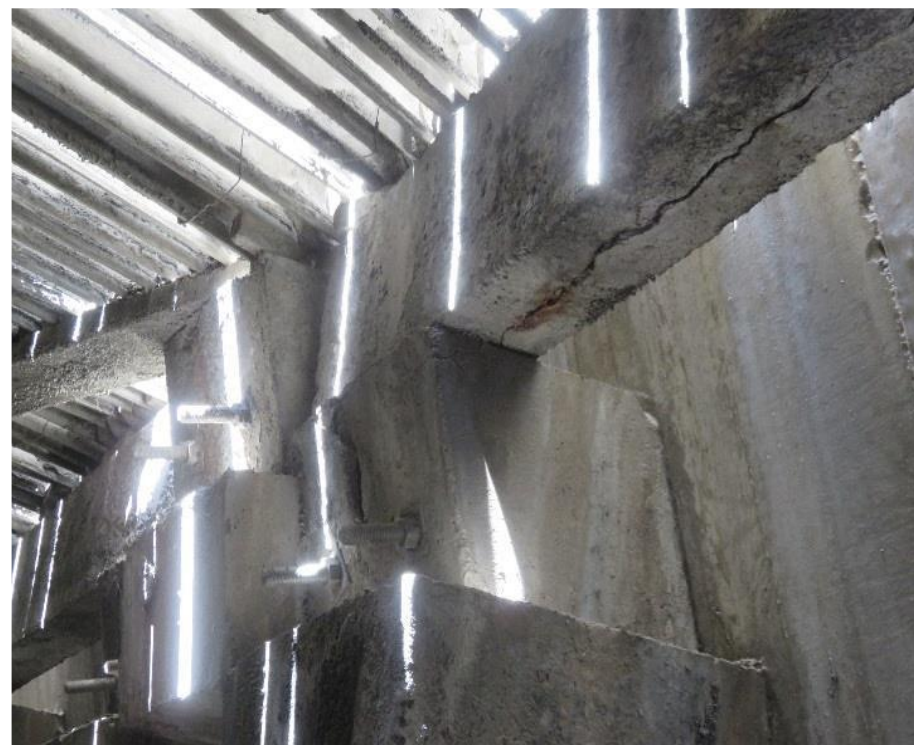
Figure 4: Ring Beam Cracking
