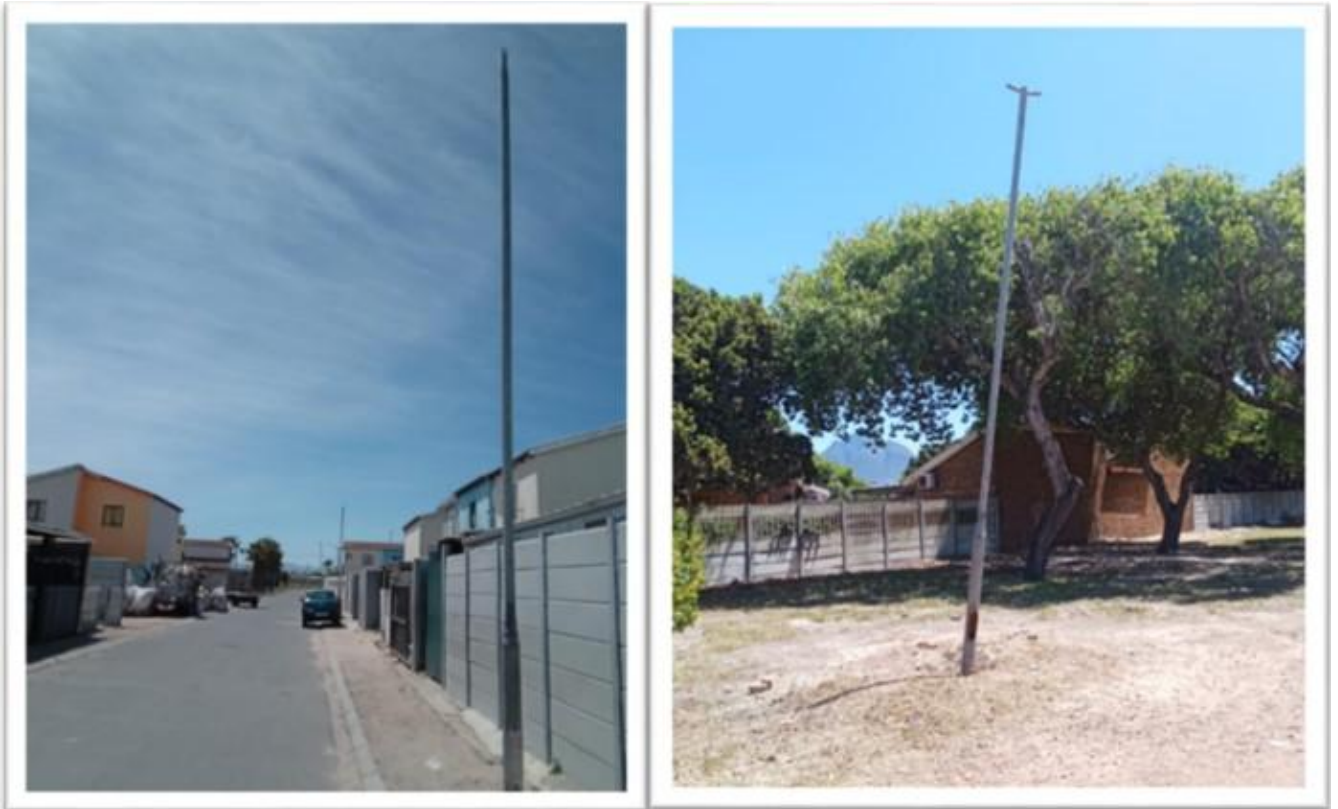
Picture 1 and 2 Luminaires Stolen
