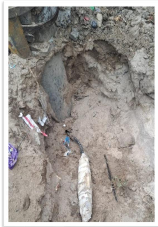
Picture 6 Streetlight Cable Stolen
