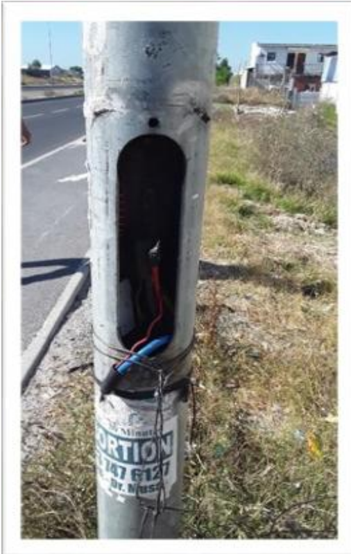
Picture 3 Pole Cover and Cables Stolen
