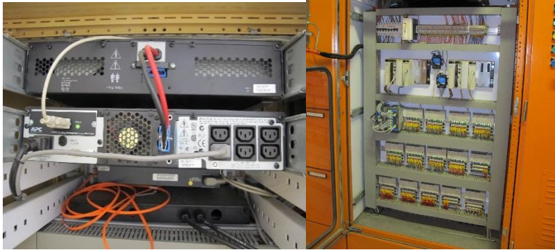
Rack mount UPS with additional battery pack
