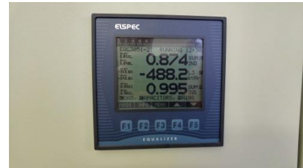
DPFC switching modules and controller
