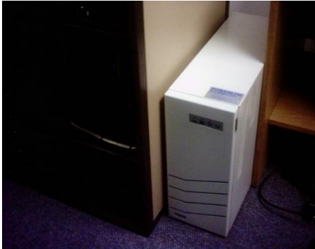
UPS in enclosed chassis mounted in MCC
