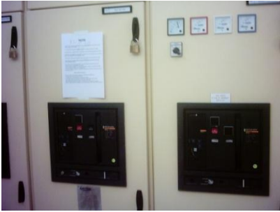
400V Incomer CB's on MCC board
