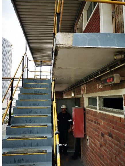
Figure 4: Damage to cantilevered walkway
