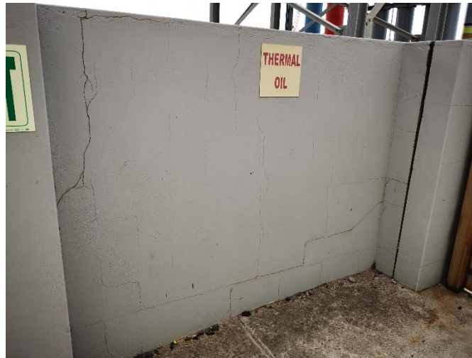
Figure 5: Cracking in boundary wall
