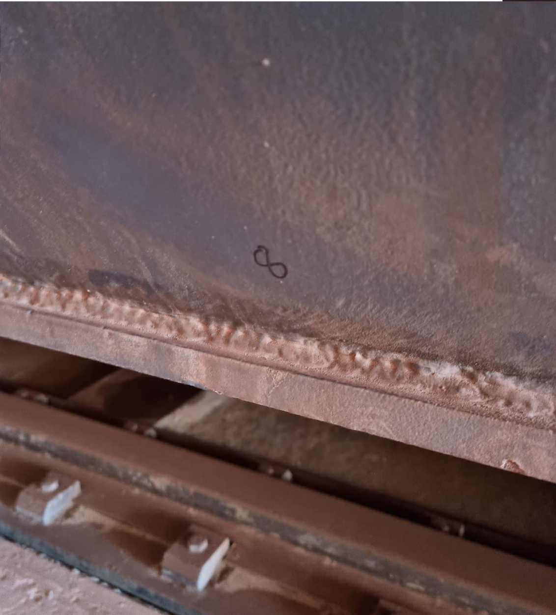
Positioner Front Pedestal Poor Quality Weld
