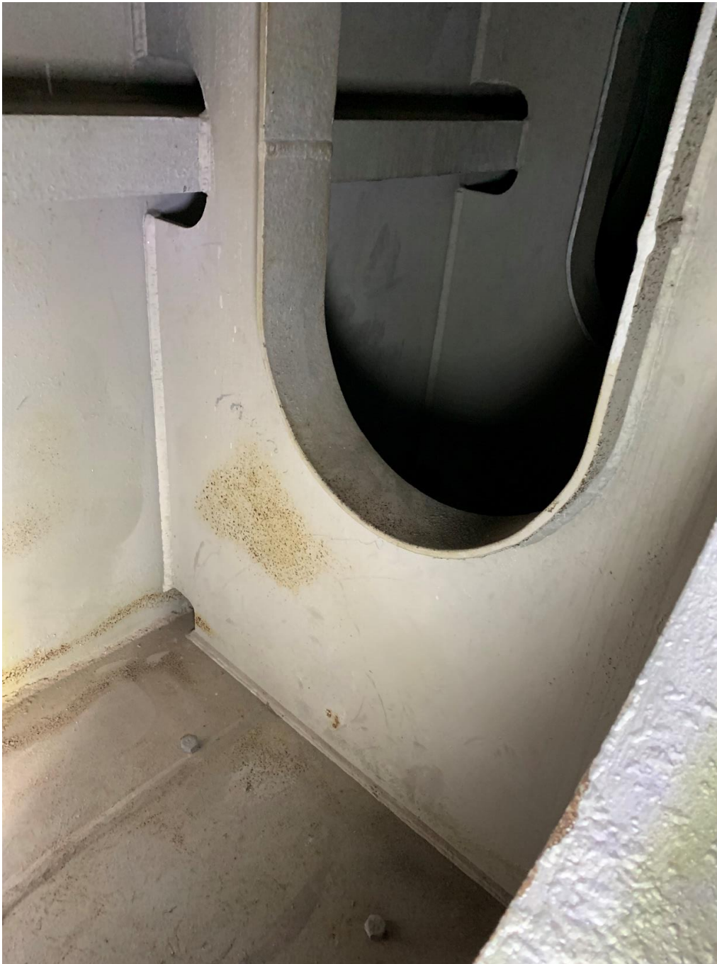
Photo 5 Tippler Rail Platform Internal Surface Corrosion
