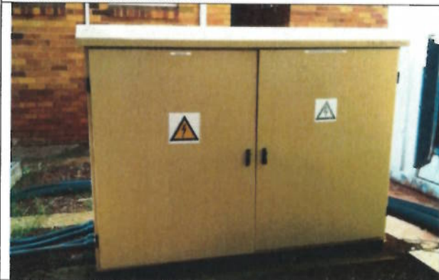
Picture 3 Distribution box
