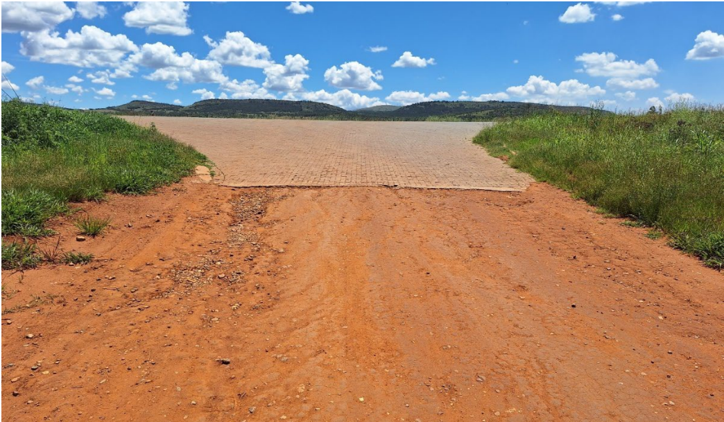
Paved bell-mouth on Western side of Gravel access road where it meets with the R550.
