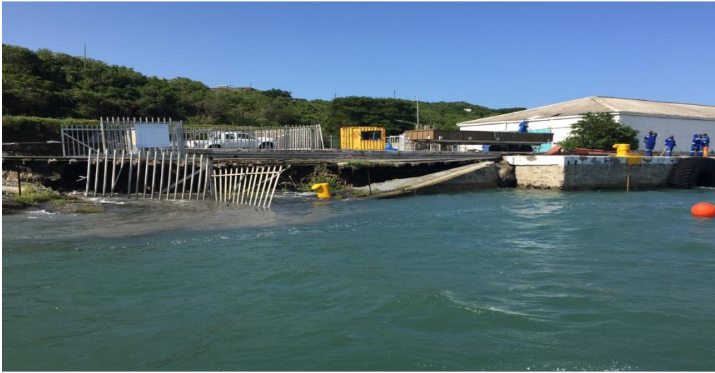
Figure 1: Collapsed section of the Quay wall.
