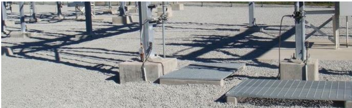
Figure 4: Substation operator grids - to be installed at selected locations (where touch voltages present a threat inside the substation and where concrete brick paving is employed).
