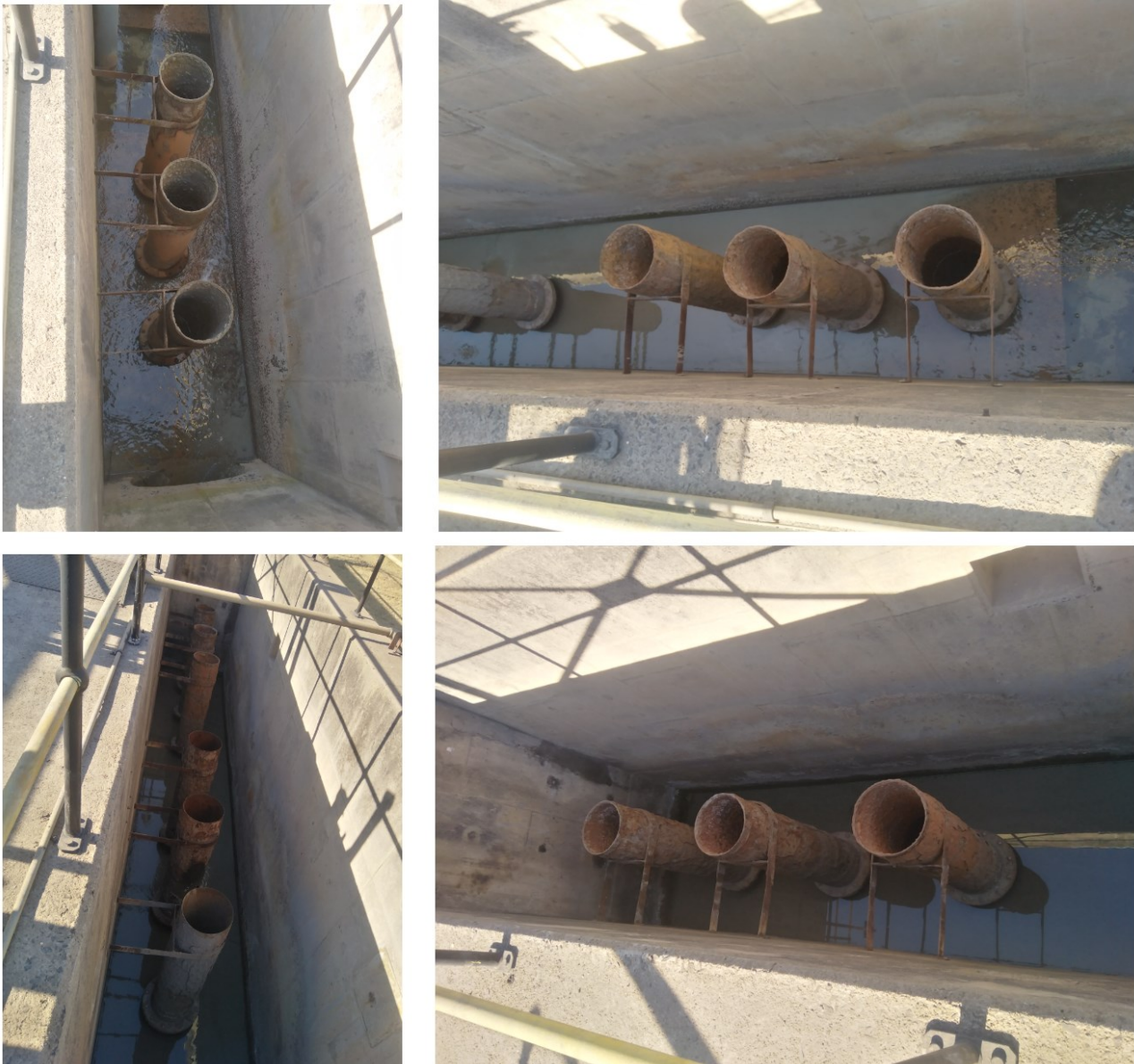
Figure 4: Clarifier separator tubes
