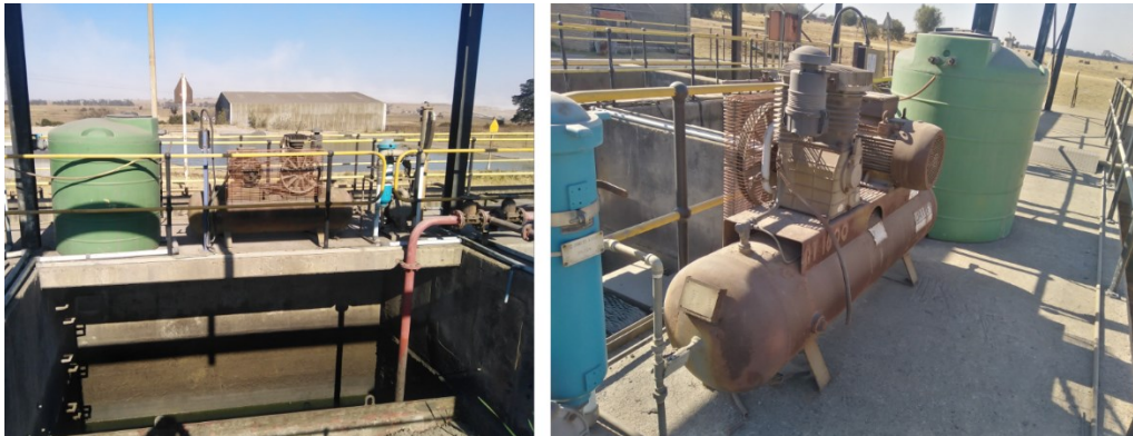
Figure 9: Oil separation compressor plant
