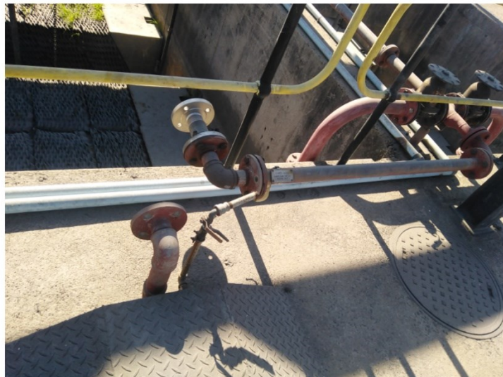
Figure 6: Clarifier discharge valve 1 and 2
