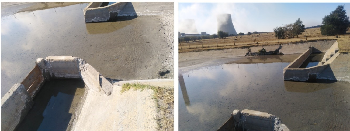
Figure 3: Sludge drying bed
