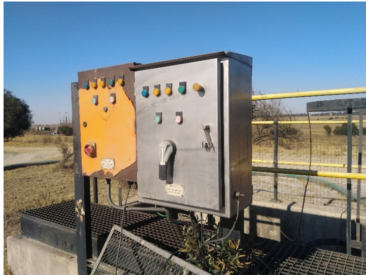
Figure 2: sludge sump local control panel
