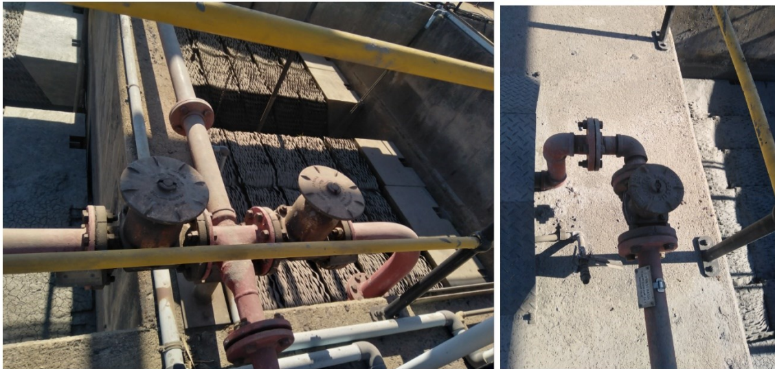
Figure 5: Clarifier discharge valve 1 and 2
