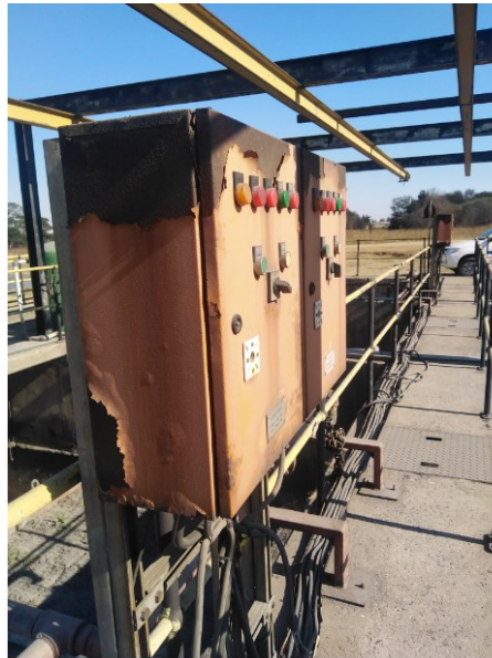
Figure 7: Clarifier local control panel
