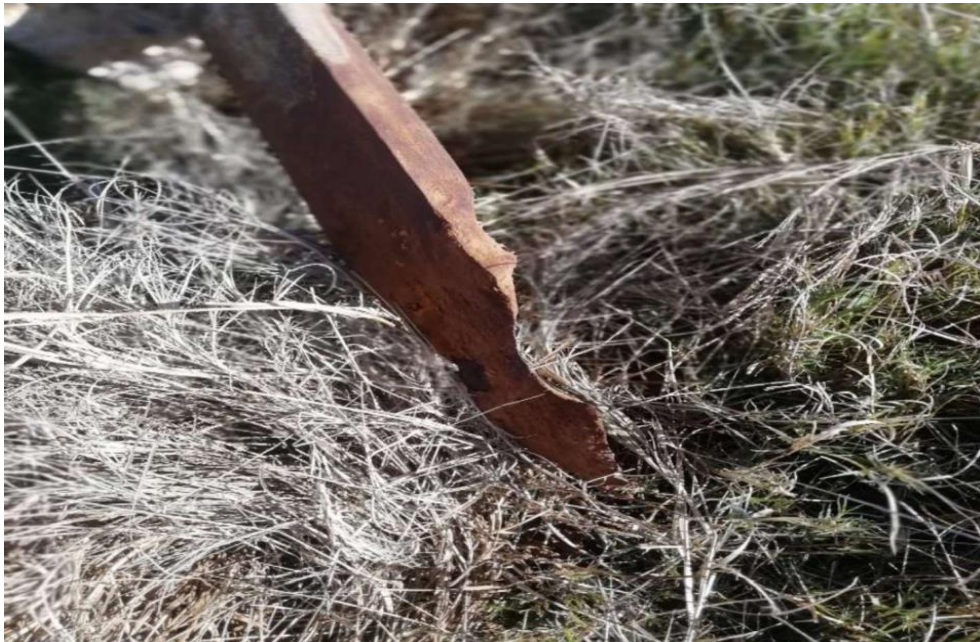
Figure 5: Corrosion of link plate
