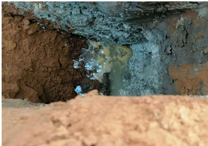
Figure 9: Water encountered in the excavation
