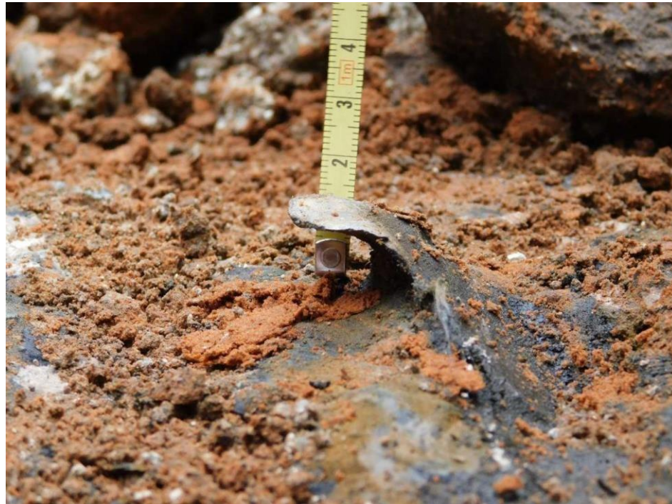
Figure 7: Breaking point of the corroded link
