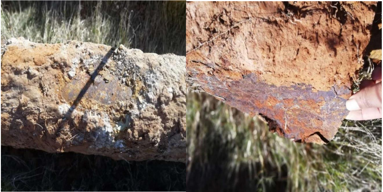
Figure 4: Corrosion on the encasement
