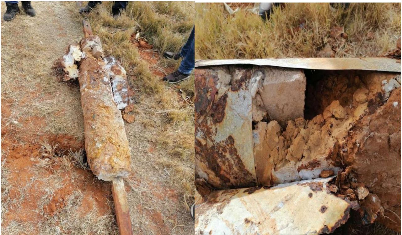
Figure 6 : Debris and bricks inside the encasement
