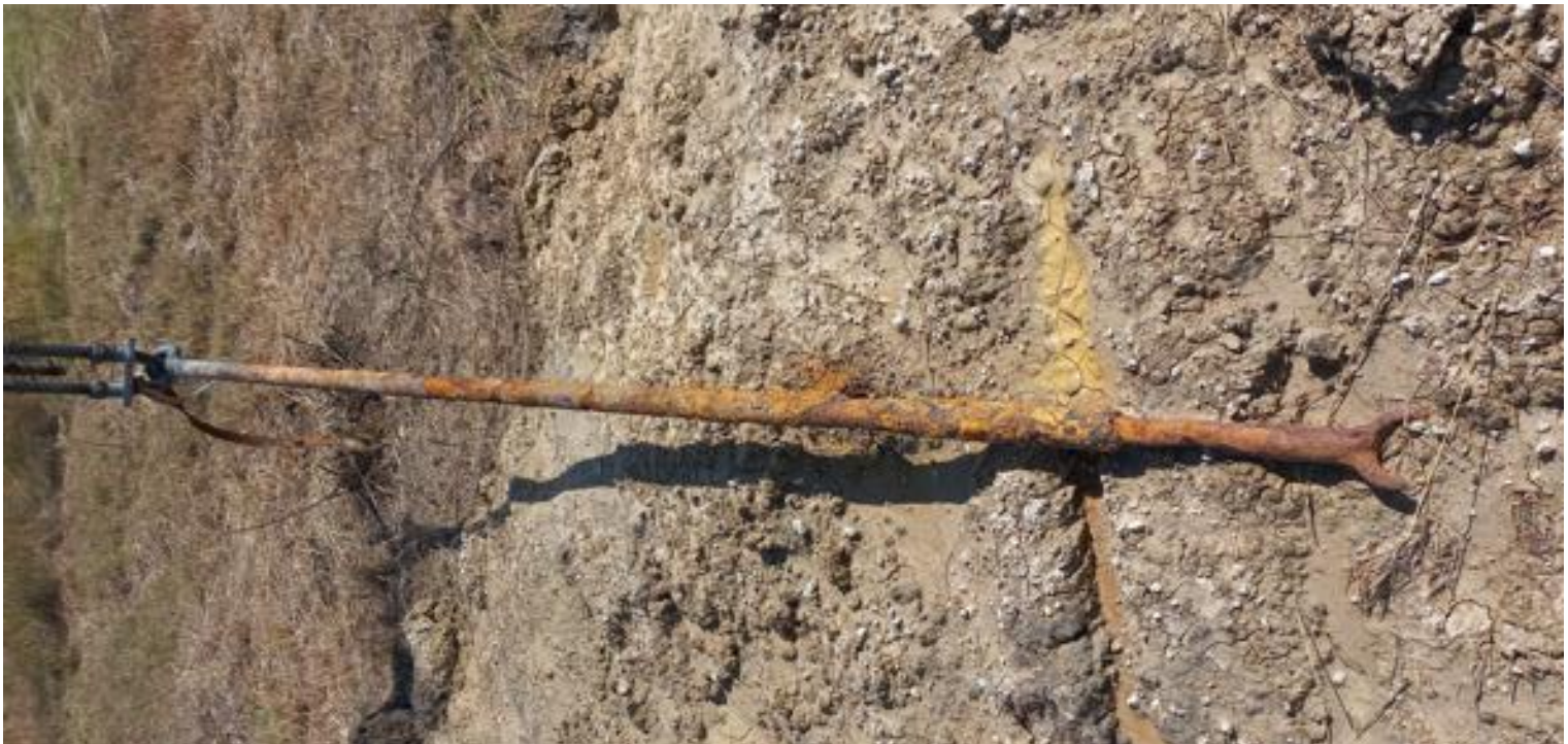
Figure 4:Failed guy anchor
