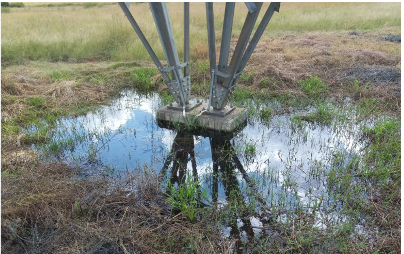
Figure 10: Ponding of water around the centre mast of tower 67
