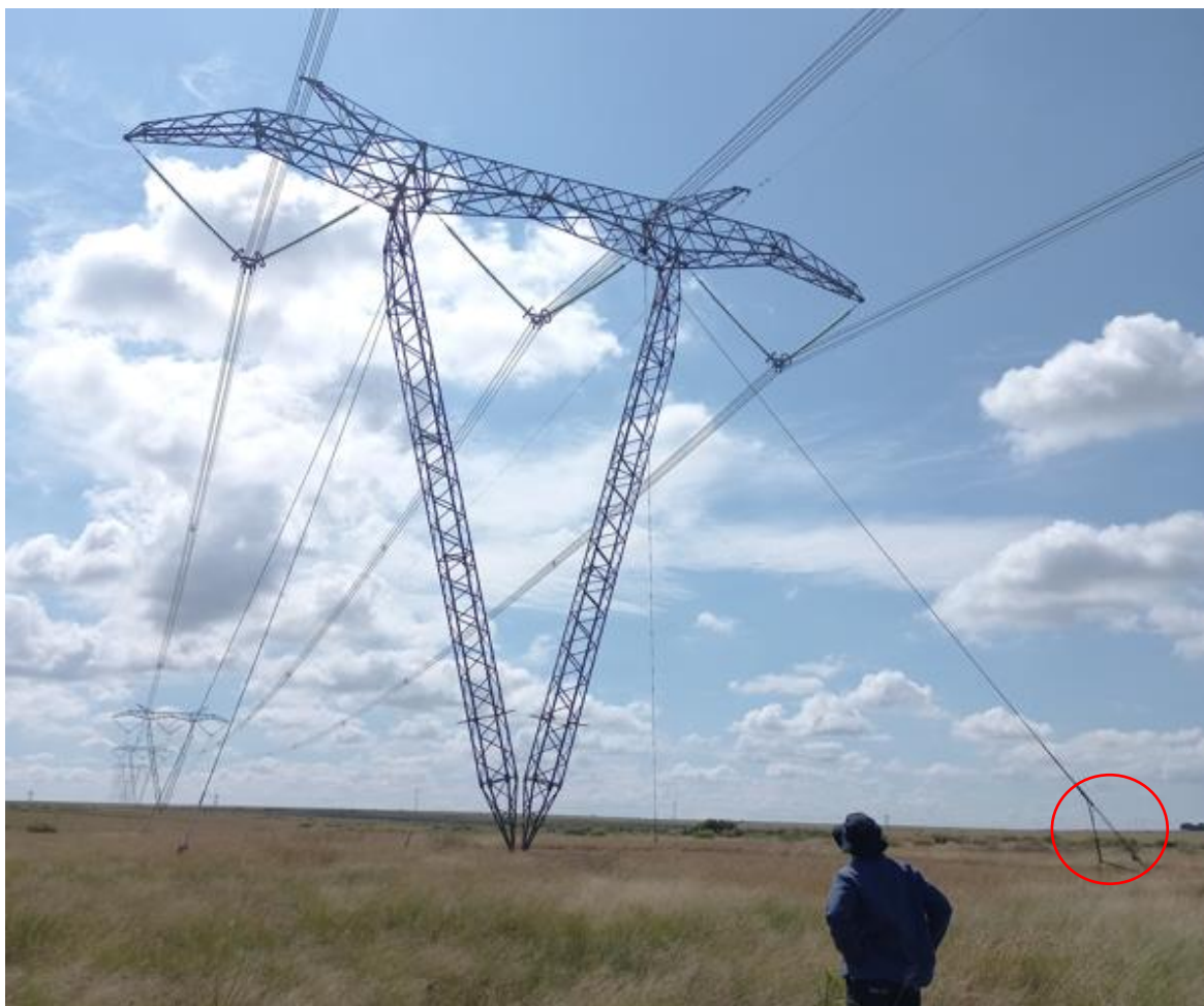
Figure 3: Tower 672 (701B) failed guy anchor
