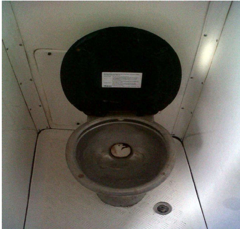
Figure 1.3 – Fixed Sceptic Toilet
