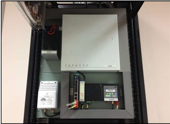
Figure 1: Example of Well Organised Security Equipment Cabinet.
