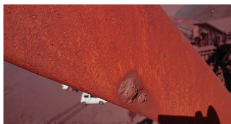
Boom upper support structure
