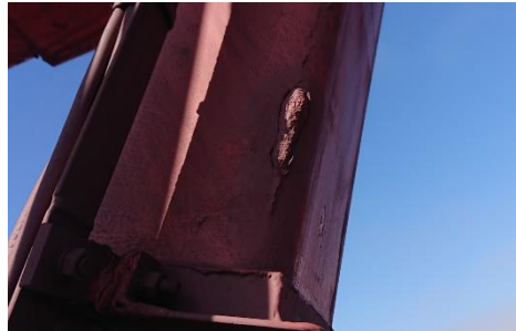
Boom upper support structure
