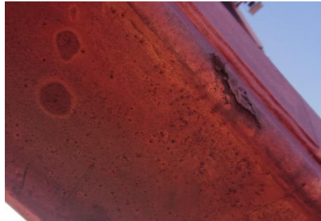
Boom upper support structure
