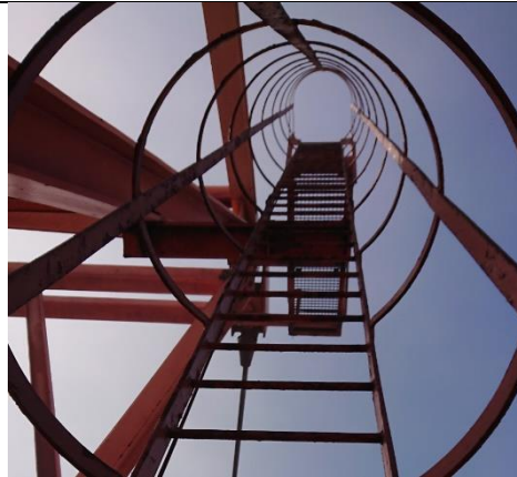
Counterweight frame catladder
