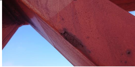
Boom upper support structure
