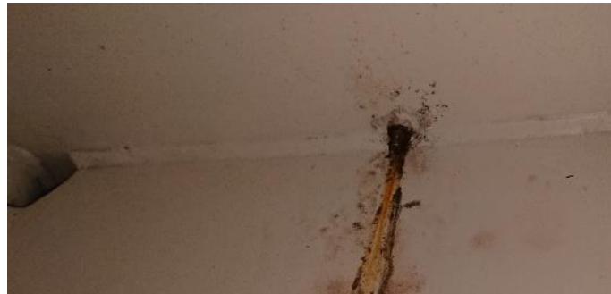
Inside slew deck – nut missing
