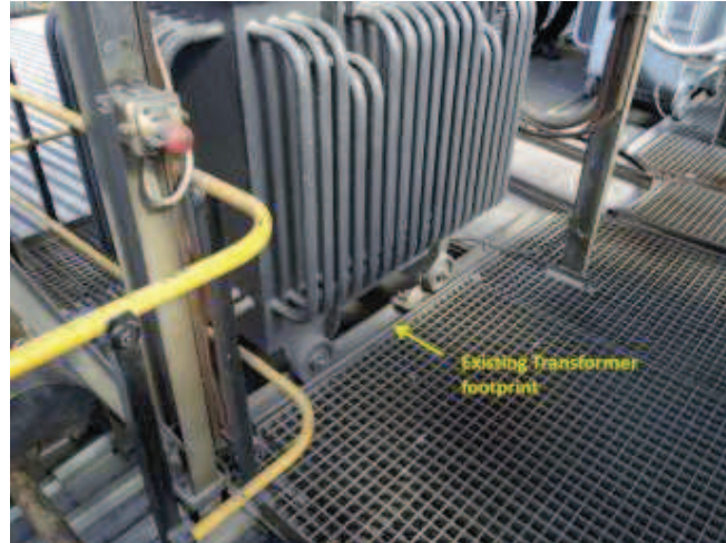
Figure 6: Existing transformer footprint
