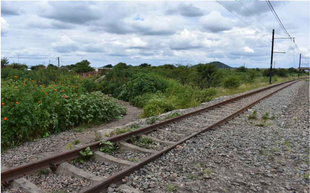
Figure 8: Bridge 8 - Illegal crossing path over rails
