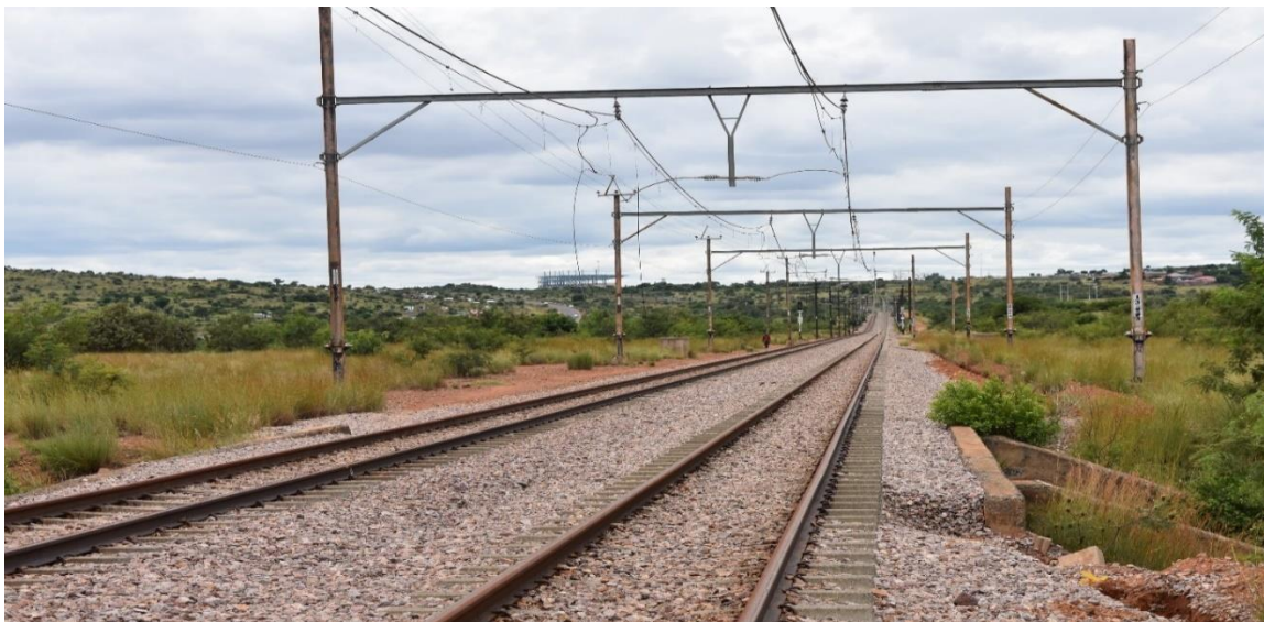
Figure 5: Bridge 2 - Damaged railway formation due to footpaths shown to the right next to culvert
