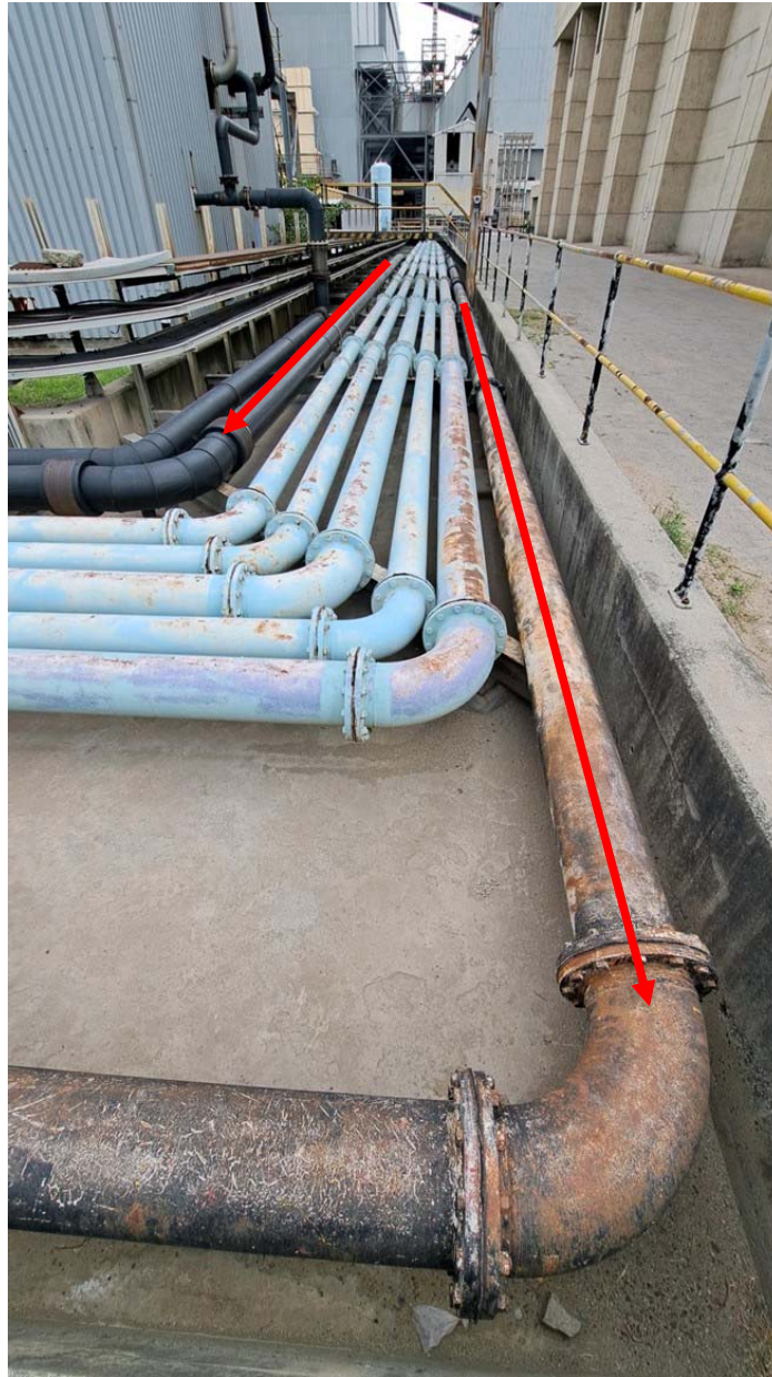
Figure 13: Chemical effluent pipes outside WTP indicated in red.
