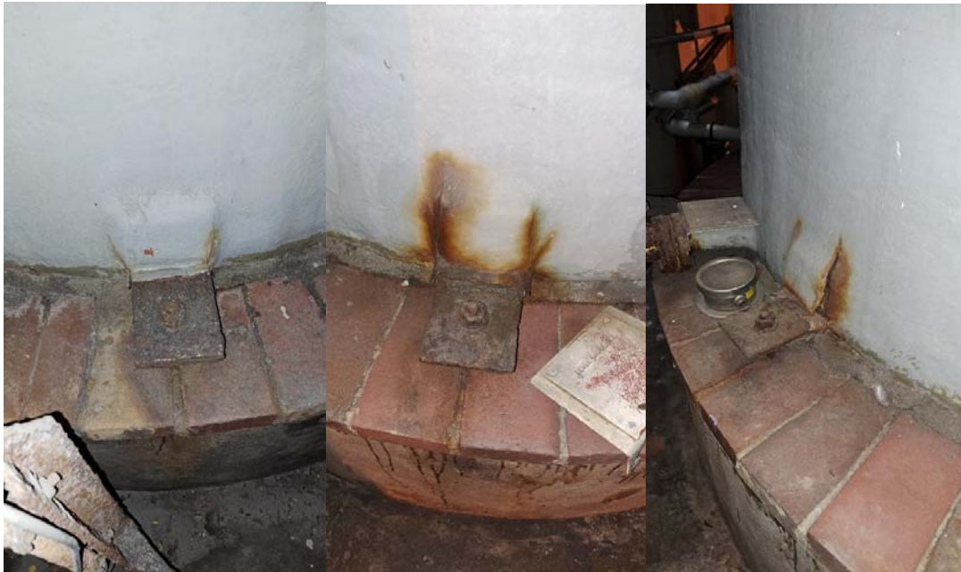
Figure 12: Current Brine measuring tank anchor lugs condition
