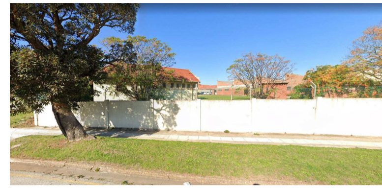
Existing diamond wiremesh fencing is not secure enough.
