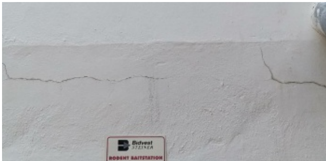
Cracks to be repaired as per surface preparations included in specification document.
