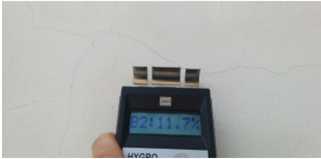
Waterproofing issues to be addressed and to conform to surface preparations as per specification document.
