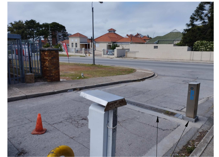
Existing security boom and floor spikes currently unused, no longer functional and redundant due to dirt ingress. Should be removed entirely as position will clash with sliding gate.
