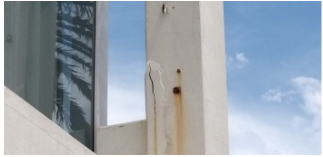
Structural failures to be addressed by structural engineer and spalling concrete to be treated as per surface preparations.
