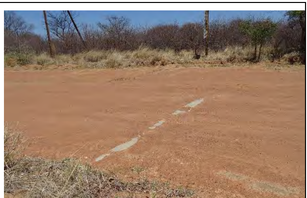
B: Top of culvert exposed on roadway
