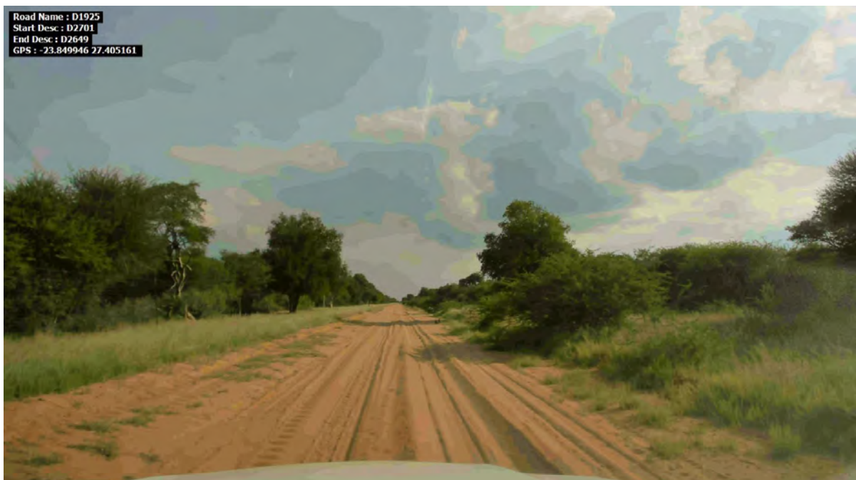
Photo 3.13: Road D1925 (km 19,8): Loose material, overgrown
