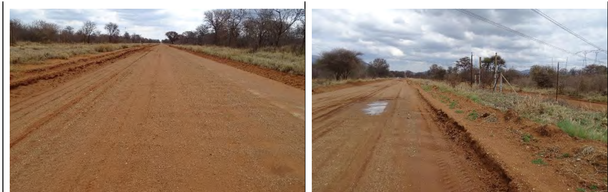
C: Corrugation on roadway
