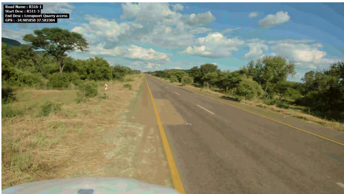
Photo 3.8: Road R516-1 (km 5,67): Crocodile cracking and pumping
