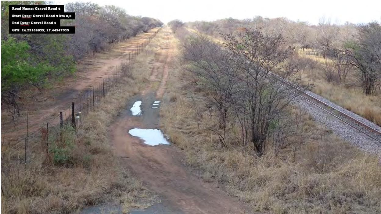
Photo 3.19: Gravel Road 4 (km 0.00) Photo taken facing the North-direction, Potholes and damage seen along roadway
