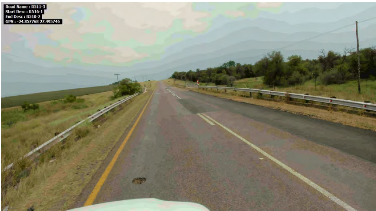
Photo 3.6: Road R511-3 (km 100,6): Surface failure in left lane and surface patches along right lane
