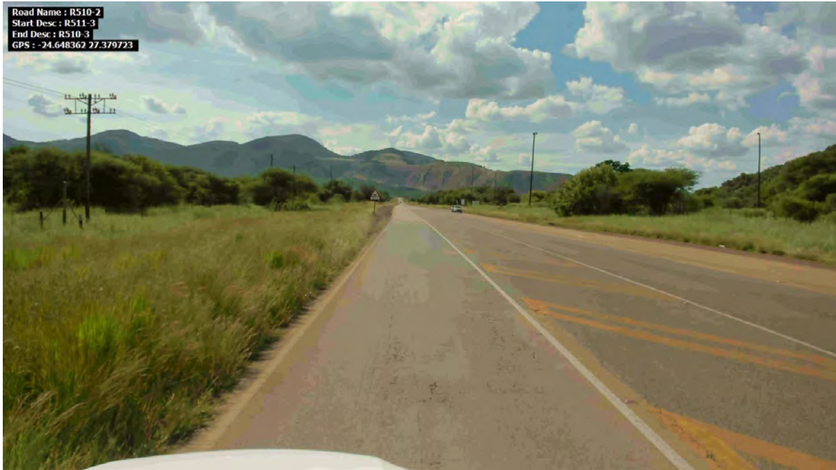
Photo 3.1: Road R510-2 (km 29,6): Surface cracks
