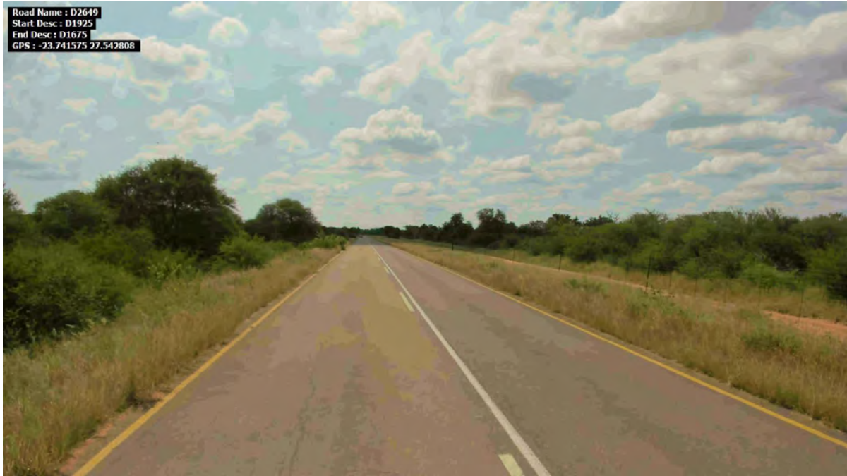
Photo 3.11: Road D2649 (km 0,15): Longitudinal crack in middle of left lane
