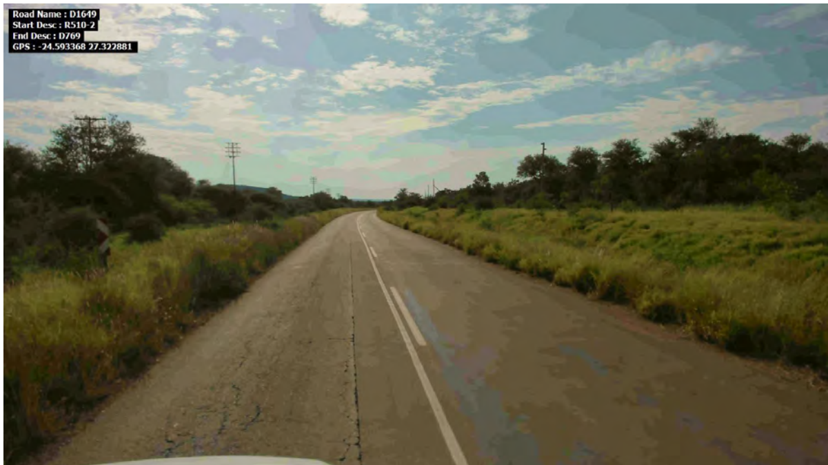
Photo 3.3: Road D1649 (km 6,88): Longitudinal crack as well as crocodile/surface cracks
