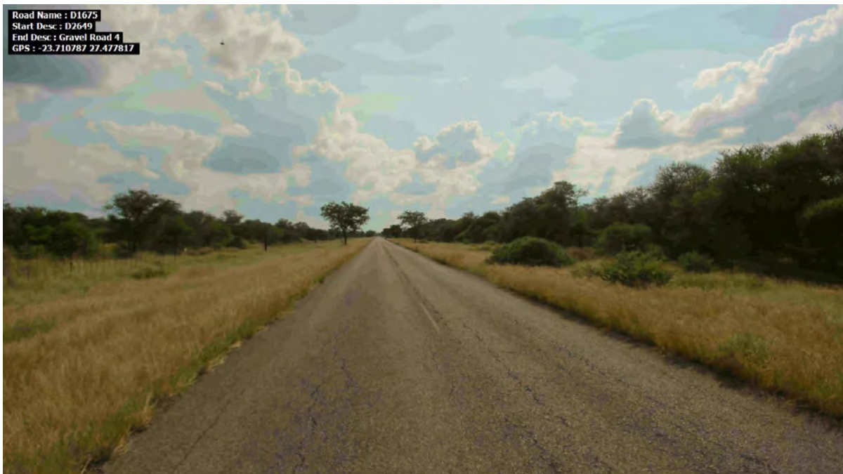
Photo 3.10: Road D1675 (km 11,6): Longitudinal cracks along seal section
