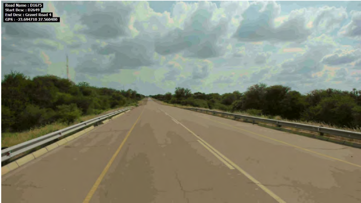
Photo 3.9: Road D1675 (km 3,0): Block cracks along asphalt section
