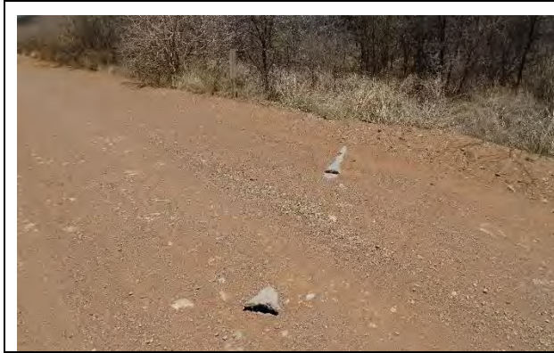
A: Top of culvert exposed and damaged on roadway
