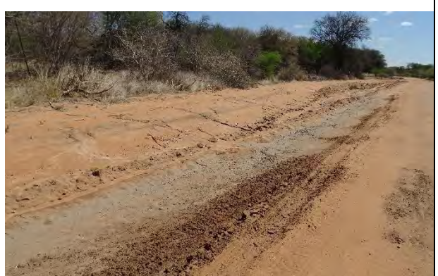
F: Roadway damaged by stormwater
