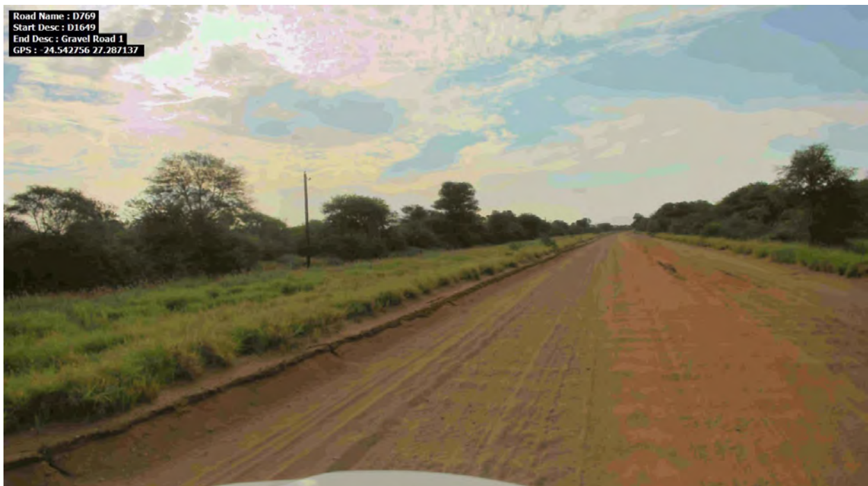
Photo 3.14: Road D769 (km 4,6): Loose material, corrugation, and windrows of gravel material along edge
