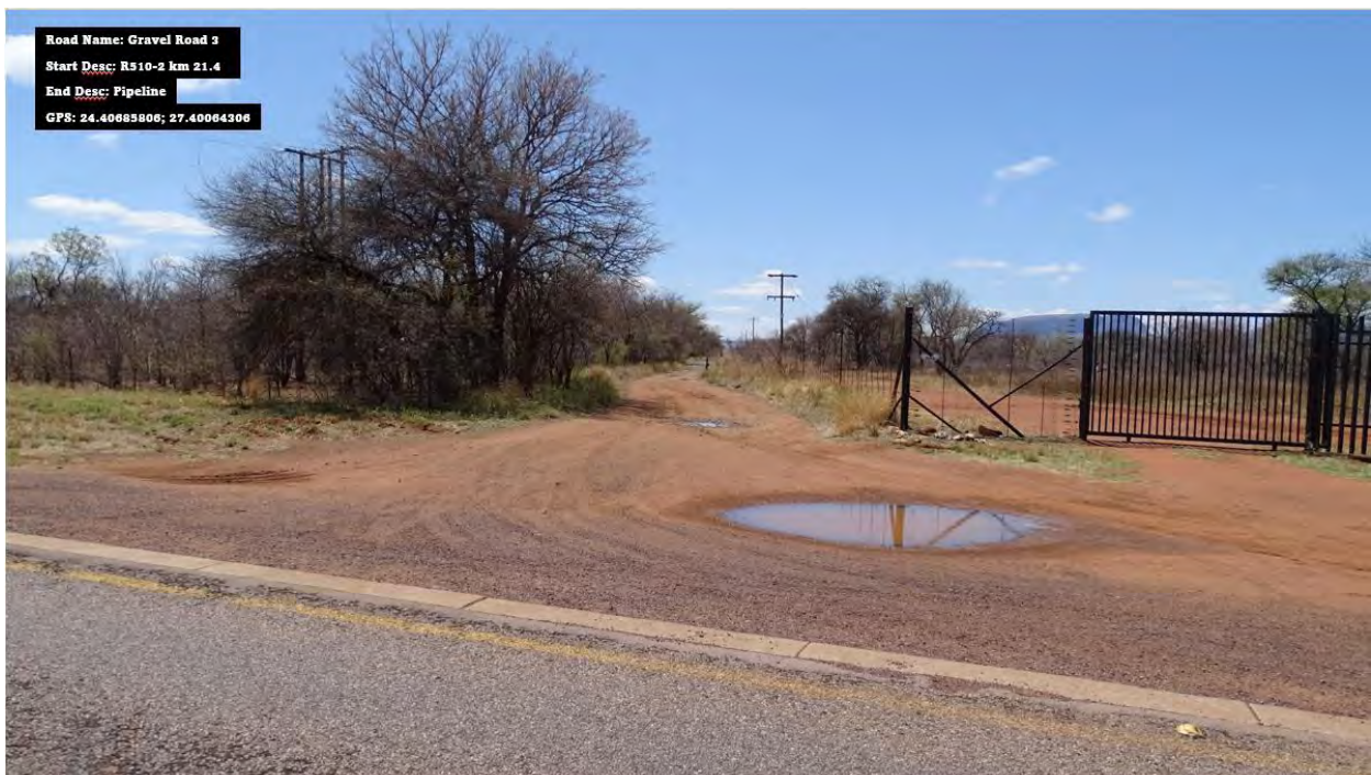
Photo 3.16: Gravel Road 3 (km 0,0): Potholes in road, narrow roadway
