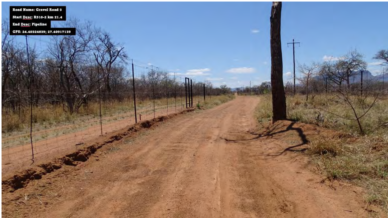
Photo 3.17: Gravel Road 3 (km 0,9): Corrugation, Narrow roadway
