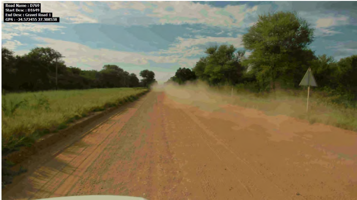
Photo 3.12: Road D769 (km 0,6): Dustiness and loose material
