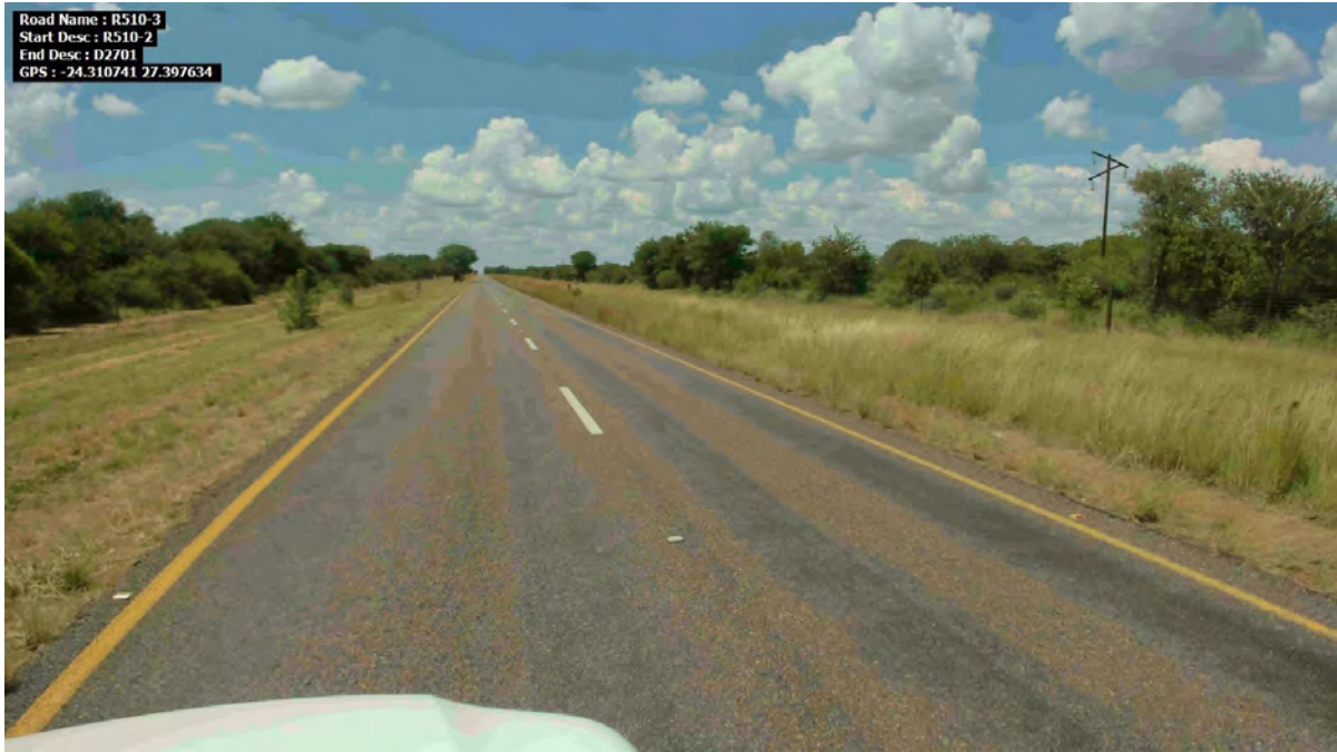
Photo 3.5: Road R510-3 (km 33,1): Flushing in wheel tracks along both lanes
