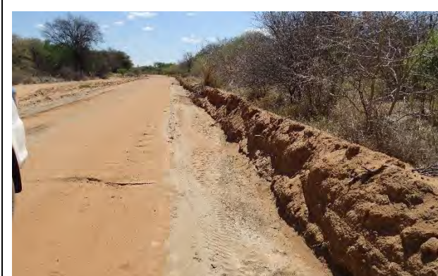
E: Windrows scoured away by stormwater
