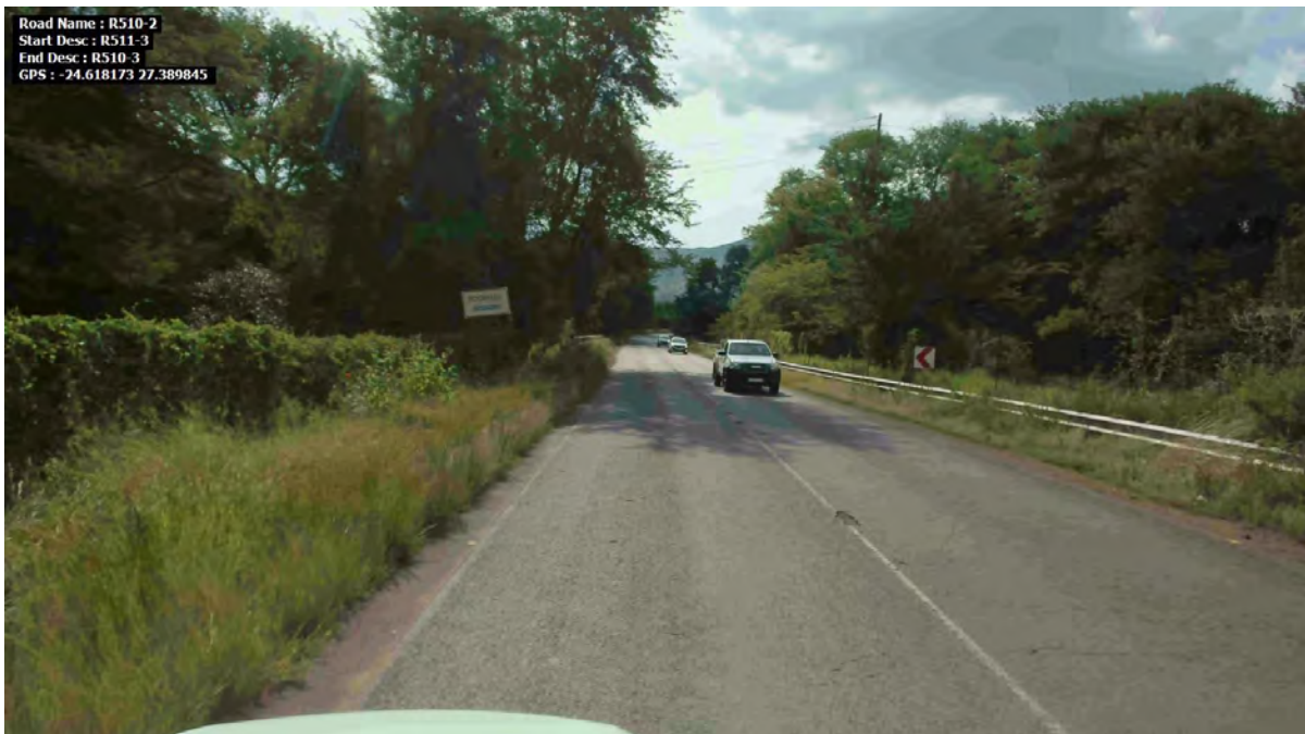
Photo 3.2: Road R510-2 (km 33,7): Surface cracks, surface failures and transverse cracks
