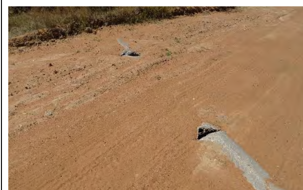
C: Top of culvert exposed and damaged on roadway
