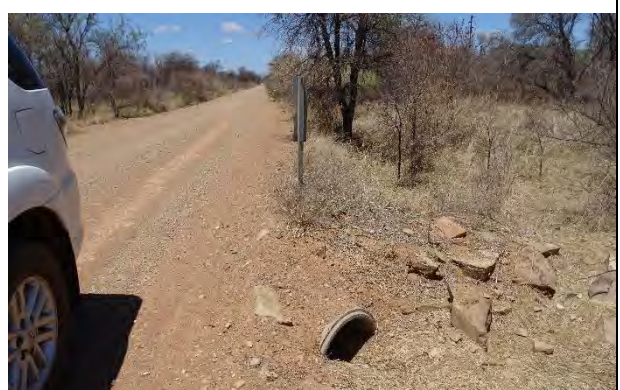
B: Blocked culvert; Little cover
