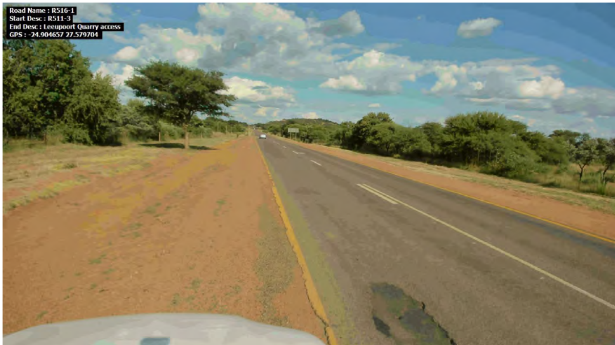
Photo 3.7: Road R516-1 (km 5,37): Surface failure and longitudinal cracks.
