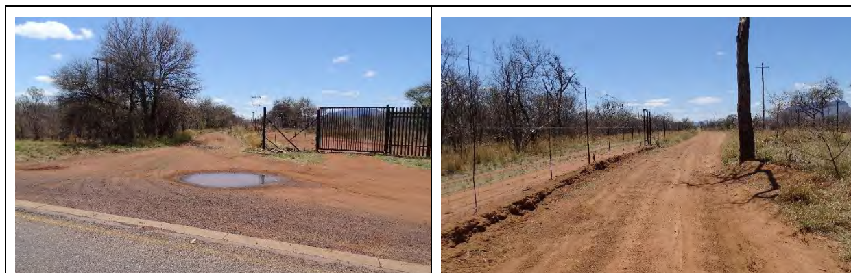
A: Entrance to Gravel Road 3; Pothole
