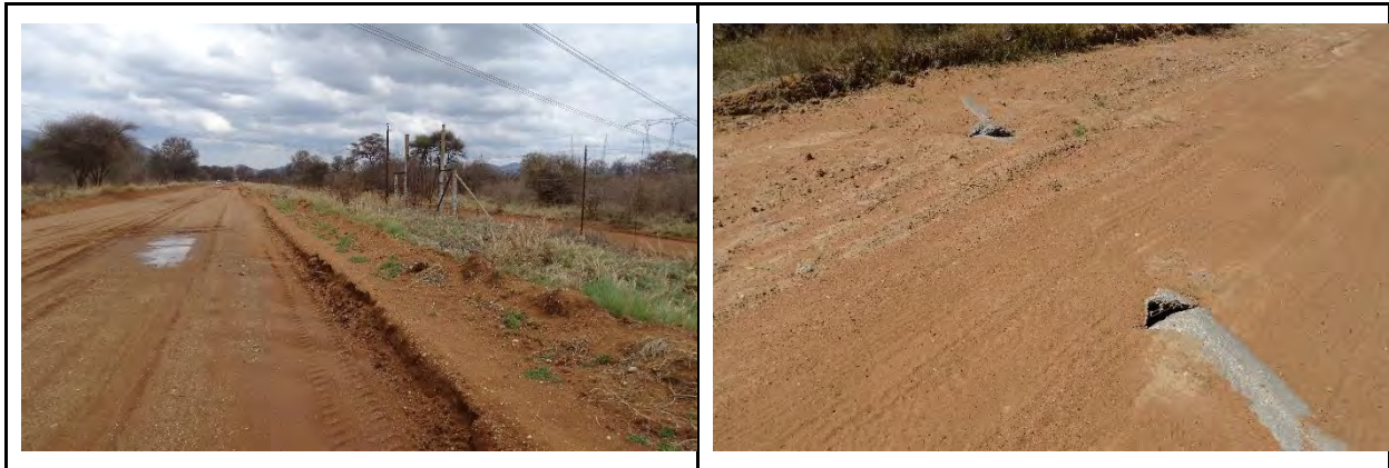
Photo 1: Ineffective drainage of roadway
