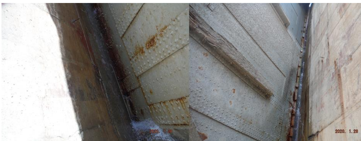
Figure 7: Leaks at Dock Gate Grooves
